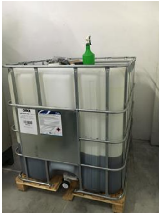
Oil tank supplying the hydraulic unit
