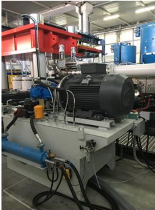
Oil-fired hydraulic unit
