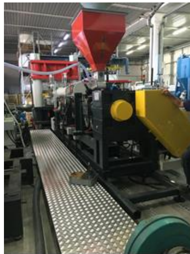
Gangway to cover electric and water cables going to the injection moulding line
