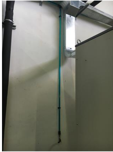
Compressed air duct for vacuum pump
